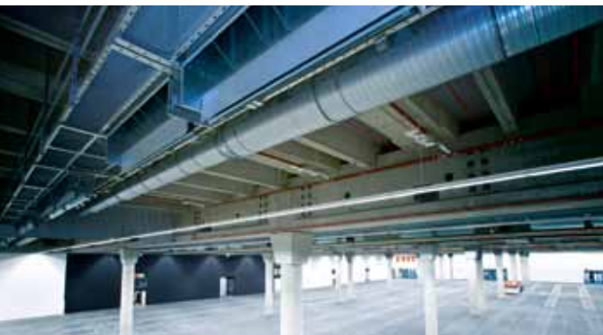
Exhibition Hall 11 in Frankfurt/Main with TROX induction units
